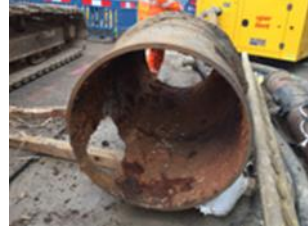
Figure 2 - Burst trunk main from the Upper Street event
