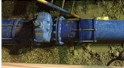
Figure 1 - Modern trunk main
